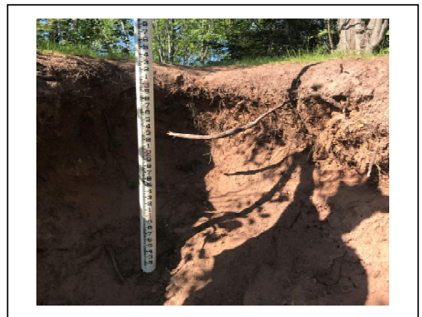
154. Island #35 – Bank erosion
