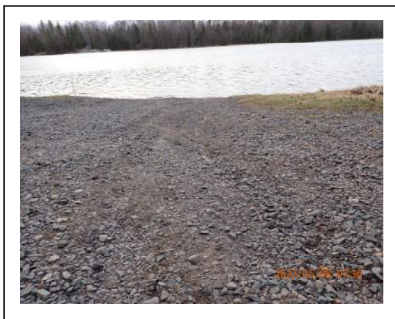
65. Sucker Hole Landing – Erosion near boat landing
