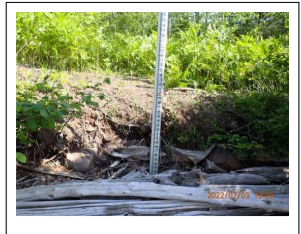
96. Island #20 – Bank erosion
